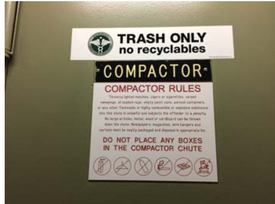
DSNY "Trash Decals" at 301 East 69 Compactor Rooms
